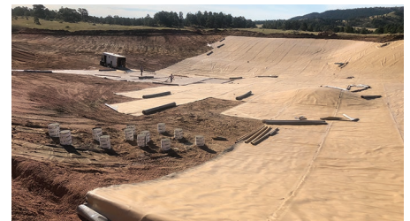
The puncture-resistant GROUNDGUARD liner was laid on the soil, with no surface preparation or underlayment required.
