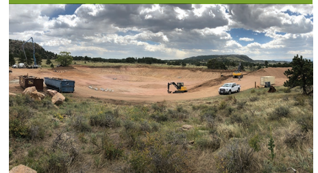
As soon as the excavation was completed, the contractor installed the GROUNDGUARD liner.
